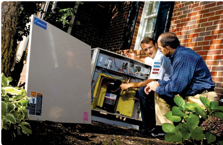
Bring your customers into the picture by helping them understand the basic operation of their comfort systems. Photo and diagrams courtesy Emerson Climate Technologies
