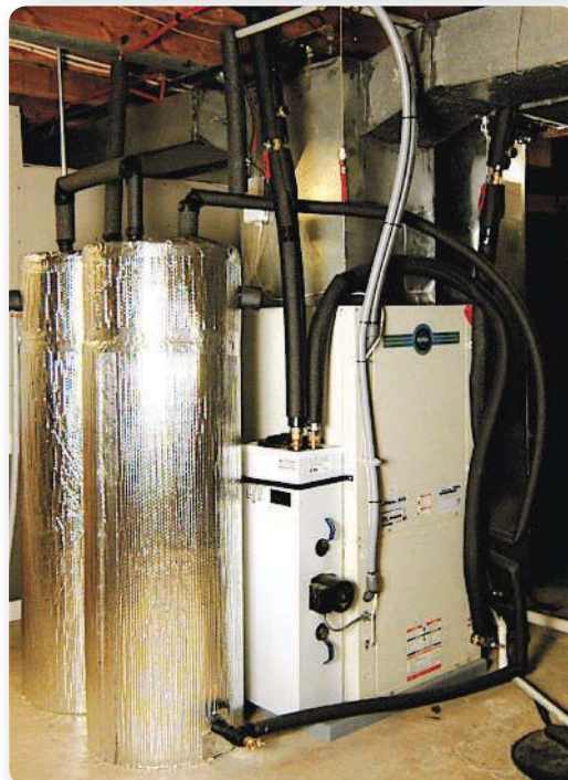
Neat installations and attention to detail, such as that shown in this geothermal heat pump installation at the Walker's home, are hallmarks of Eric Kjelshus' work.
