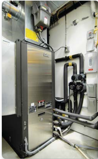
The work done by Professional Geothermal Systems drew raves from HVAC industry insiders.
