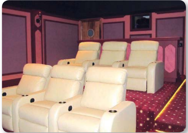
Larger grilles and ductwork ensured quiet comfort in the 'super-cool' home theater.
