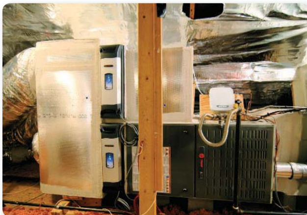
Trane's 10-year warranty was supplemented by General Air Conditioning's 4-Star Maintenance Agreement.
