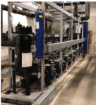
Refrigeration rack. Photo credit: Duquette.
