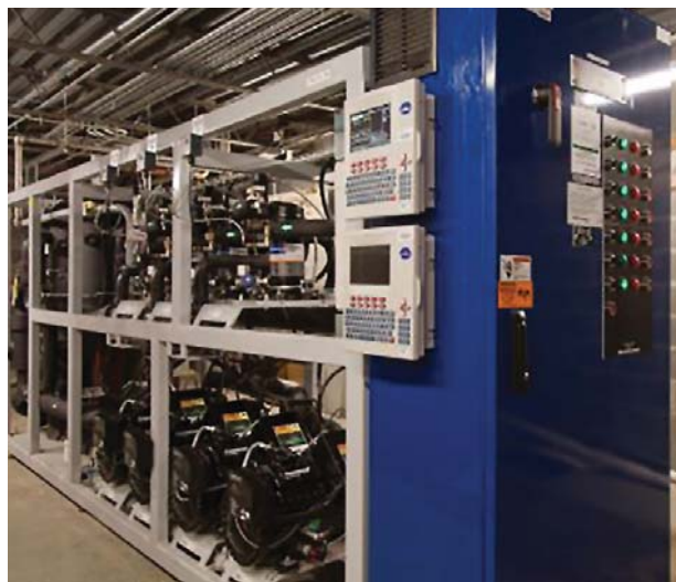
Hillphoenix, CO2 Booster Transcritical with Emerson Compression and Controls. Emerson
