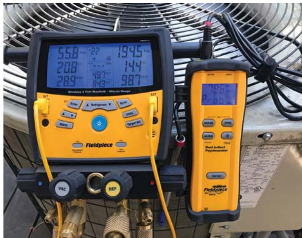
Photo 1: Measure superheat and subcooling together to "see" the refrigerant state in the evaporator and condenser. NCI
