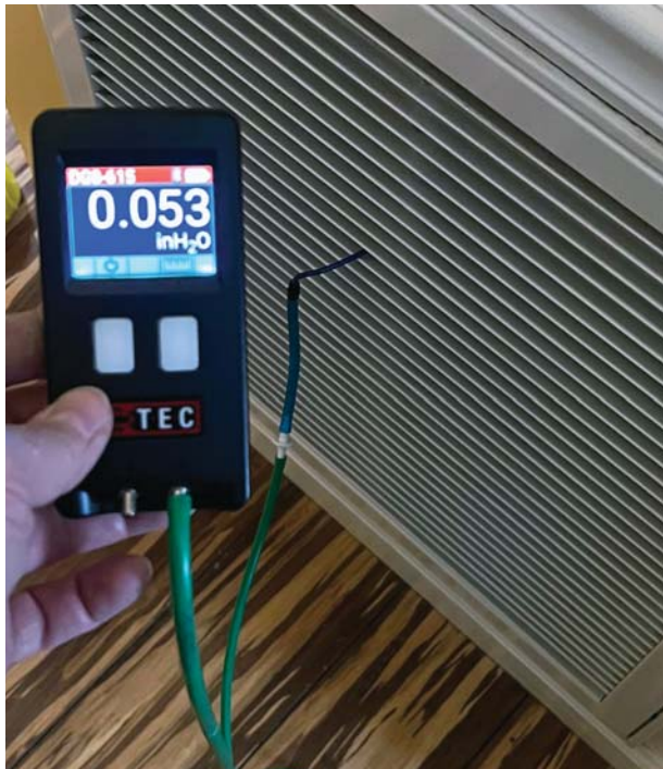
Measuring the return air filter grille pressure drop reveals much about the filter's condition. Pressure drops that look too good to be true can indicate a bigger problem, such as duct leakage.
