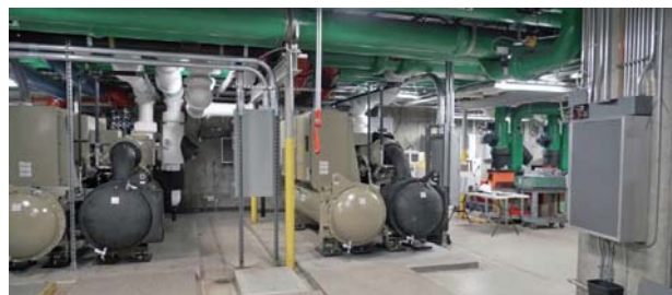
Mechanical room for the SAP Center's refrigeration system.
