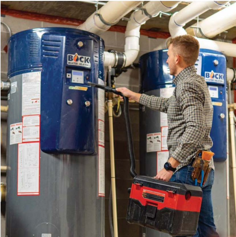
Superior training, such as NATE certification, along with the right tools and expertise allows F29 Master mechanical contractor George Heiman of Green Home Services to supply high-quality technical services for consumer and commercial HVACR equipment.
